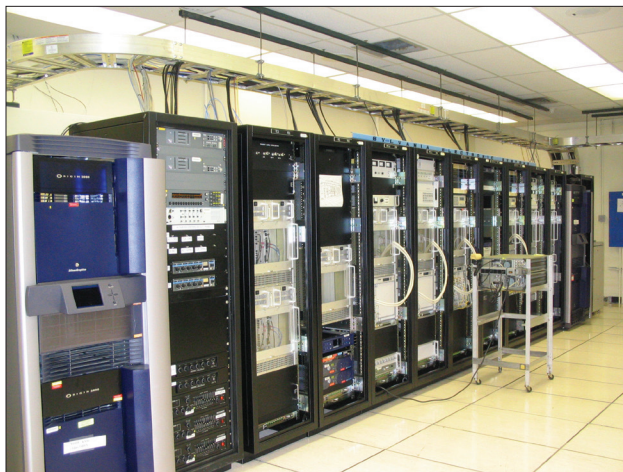
FIGURE 16. Reduced complexity and reduced costs were realized by having a common set of eleven racks for each radar.
